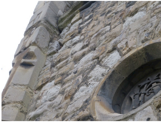
Weathering back of ragstone at the west end of the south elevation. Much past repair in cement.
