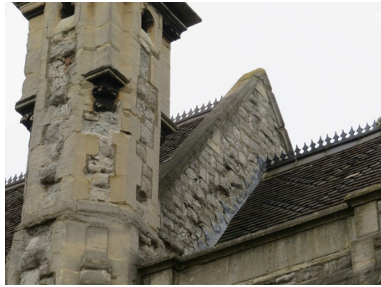
A further area of concern above the abutment of the chancel roof with that of the nave.
