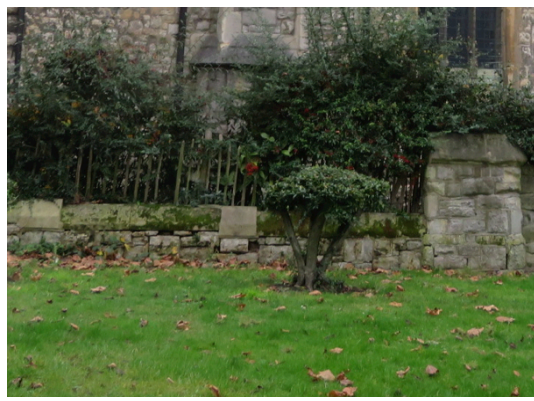
Repairs required to the south boundary wall.
