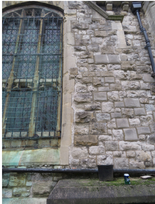
Cracking has recurred beside the garden room window.
