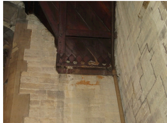
Signs of possible damp penetration below this complicated area.
