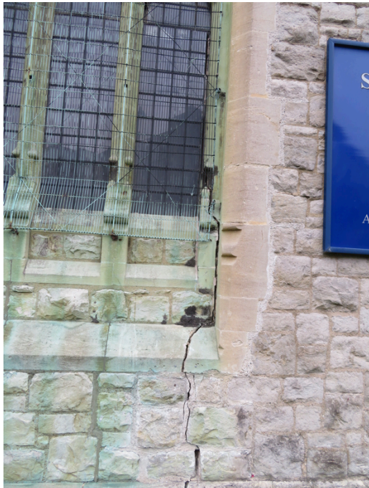
Cracking and damage the west window of the former choir vestry now requires repair.
