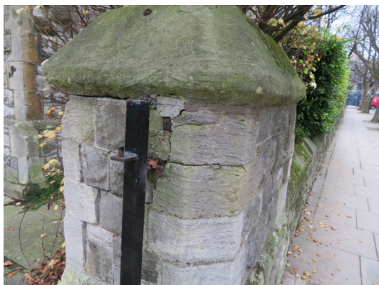
Cracking in the north east gate pier.
